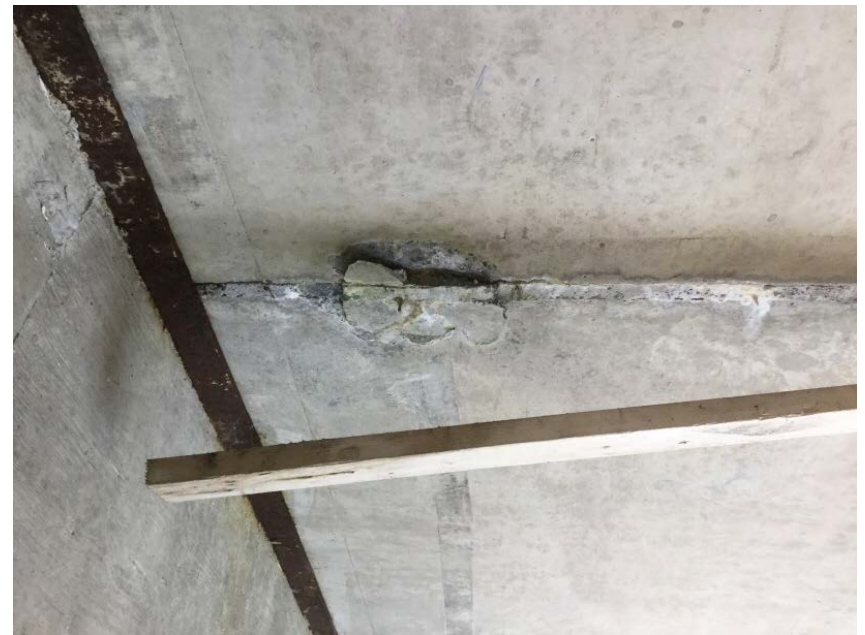
Small spall in 2 Panels - underneath
