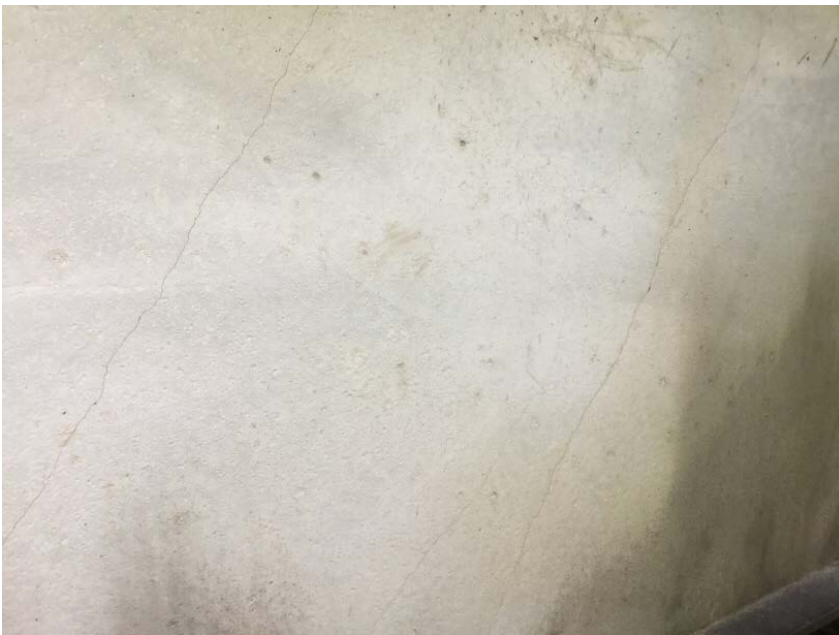
Cracking on upstream girder - minimal gap in all cracks
